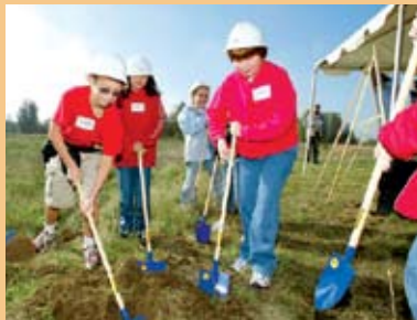
Third graders from Clatskanie Elementary school help break ground for the new Port Westward Power Plant.
